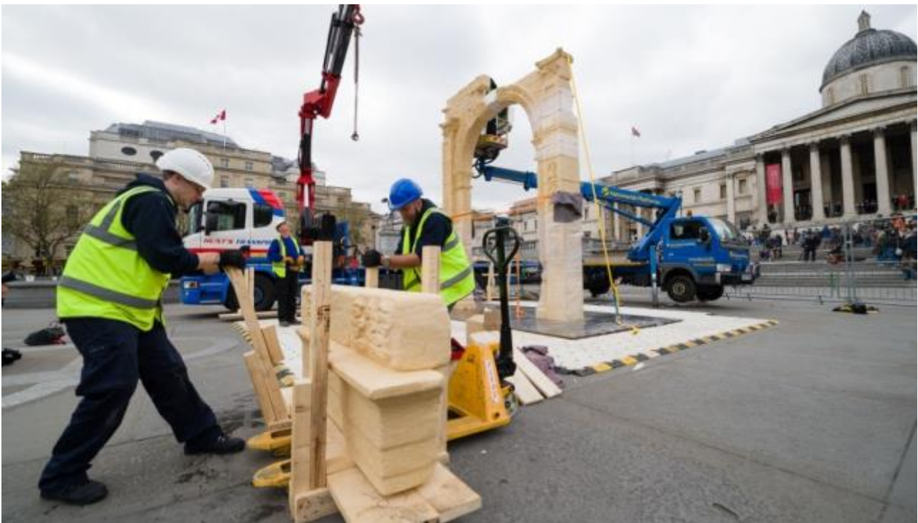
Components of the 3D Printed (and CNC milled) Palmyra's Arch replica being assembled in London
